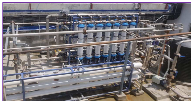
3-Stage Reverse Osmosis (RO)
