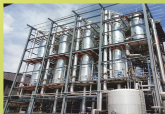
PSC Starch (Thailand) Integrated Evaporation Plant
