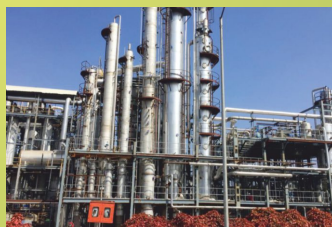
Hermes (Karnataka) - ENA Plant With Evaporation
