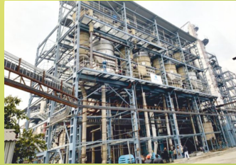
P T Molindo Raya (Indonesia) Evaporation
