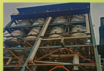
Vilas SSK, Maharashtra - Evaporation Plant
