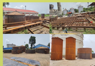
KRIBHCO Green Energy, Gujarat Grain Distillery
