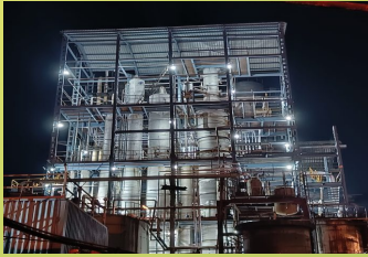
KM Sugars Ltd Uttar Pradesh ENA Plant
