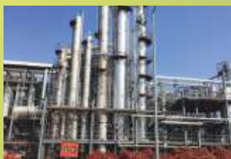
Hermes (Karnataka) - ENA Plant With Evaporation
