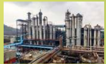
Shamnur Sugars Ltd, Karnataka EPC Grain/Molasses Distillery, Slop Co - Generation & ZLD
