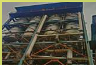
Vilas SSK, Maharashtra - Evaporation Plant
