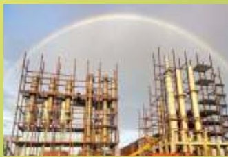
Shri Basaveshwara, Karnataka EPC Molasses Distillery, Slop Co- Generation & ZLD
