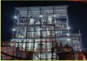
KM Sugars Ltd Uttar Pradesh ENA Plant
