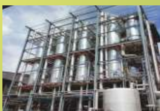
PSC Starch (Thailand) Integrated Evaporation Plant
