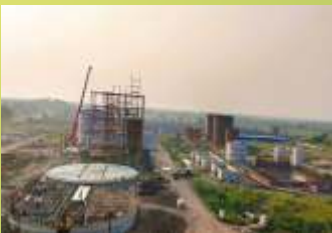
Edhas Biofuel Refinery Industries Pvt. Ltd., Gujarat- Grain Distillery
