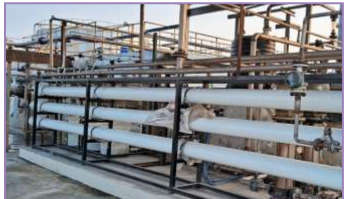
"ER-max" Water & Waste Water (ZLD) system.
