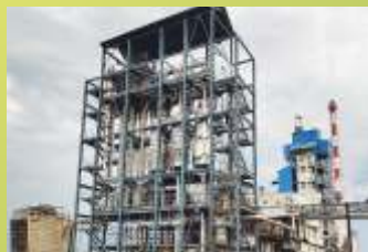
EID Parry (Andhra Pradesh) Evaporation Plant
