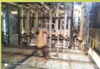
Bajaj Hindustan (UP) Wash To ENA Distillery Modernisation
